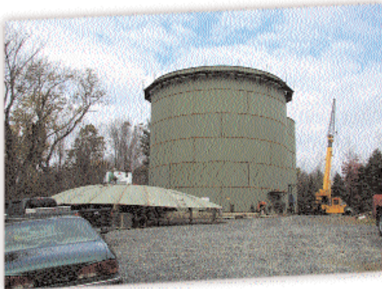
KJ's two water tanks (when under construction), which aid the groundwater wells in dealing with peak and off-peak demand.
